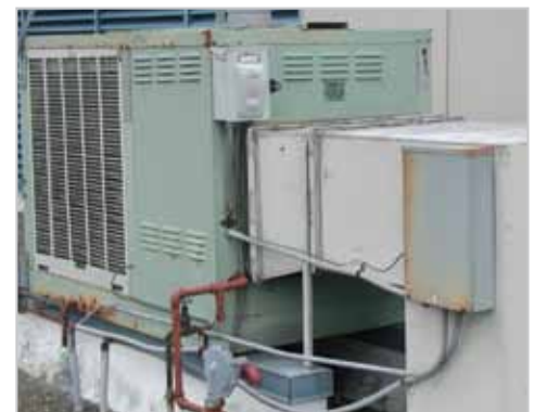
Ameresco upgraded HVAC systems and failing equipment, such as these.
